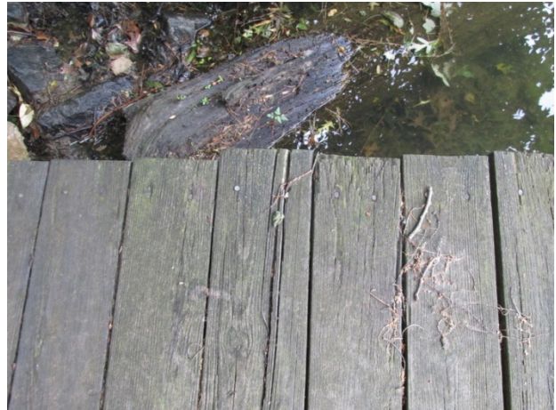
Split board at dock
