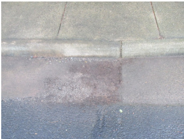
Concrete curb and gutter settlement
