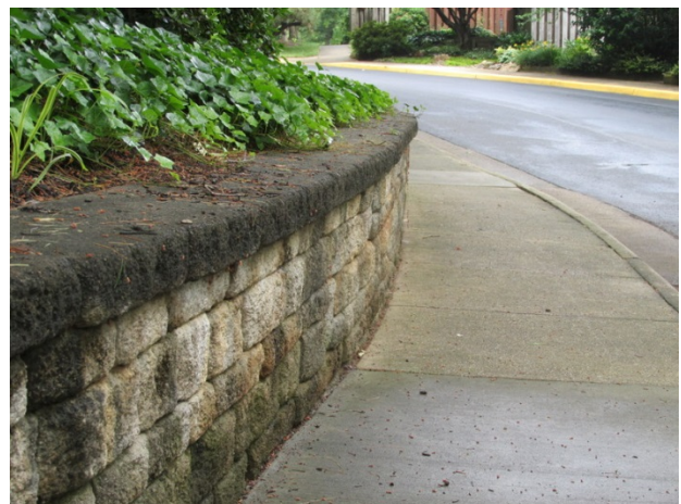
Retaining wall lean
