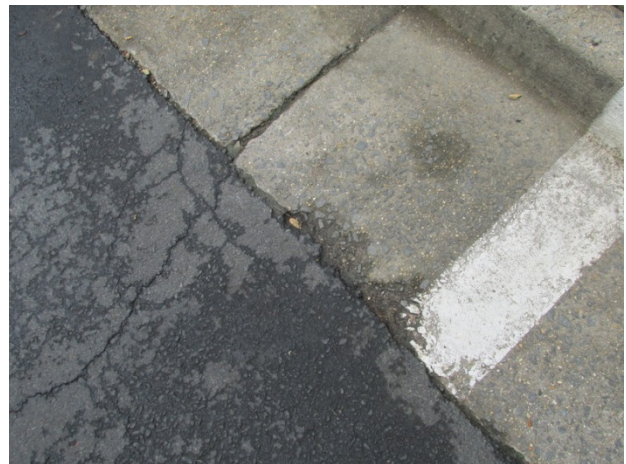
Curb and gutter damage
